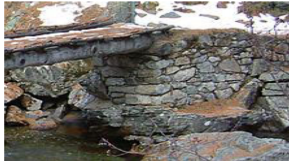
Dry set masonry supports a rustic log bridge, where it provides a well - drained support for the log (which will increase its service life)
